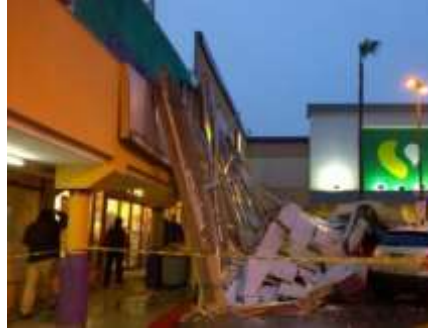
Figura 1.6 Espectacular colapsado, centro comercial de Baja California ( http://zetatijuana.com/2017/02/reportan-danos-por-vientos/ )
