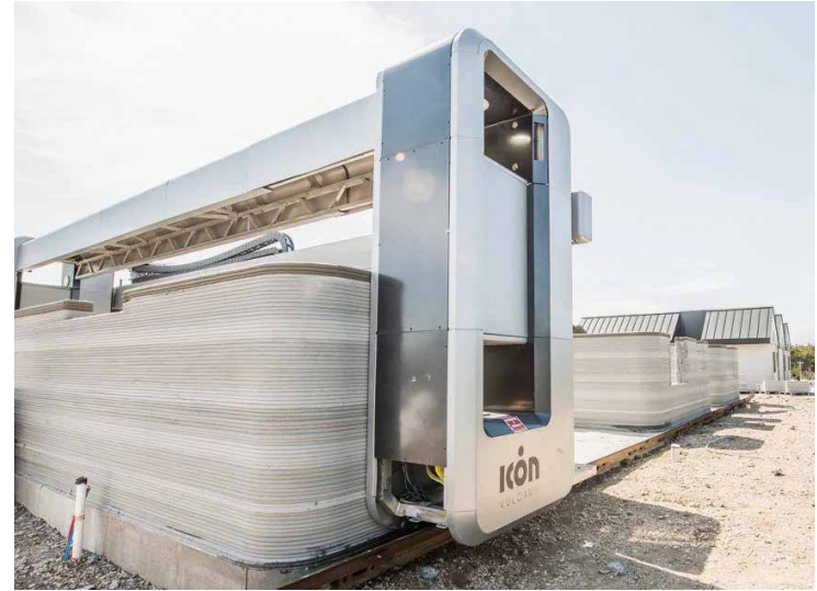
Figura 80. Icon imprime casas en 3D usando su impresora Vulcan. Fotografía de Regan Morton, 2021, ( https://metropolismag.com/viewpoints/3d-printing-is-speeding-up-the-automation-of-construction/ )
