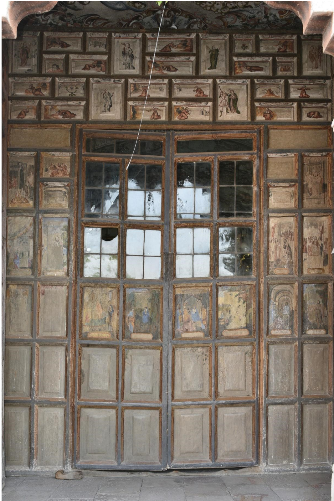
Fig.4. External view of the central structure of the cancel at the entrance door of the Sanctuary of Jesus the Nazarene, Atotonilco, near San Miguel de Allende, México. Photo provided by Ana María Pimentel.
