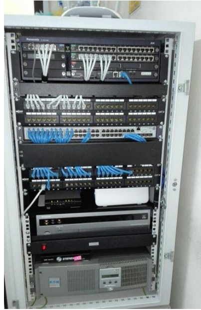
Fig. 4.10 Gabinete y Access Point de Metro 2
