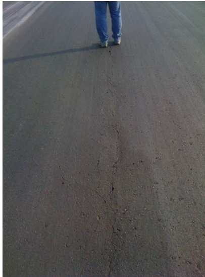
GRIETA LONGITUDINAL MAYOR A 3 mm
