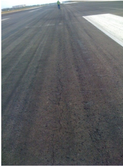
GRIETA LONGITUDINAL MAYOR A 3 mm
