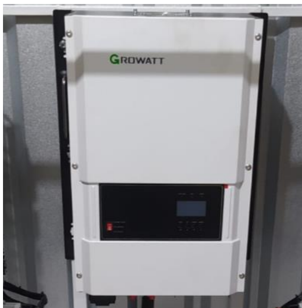
Figura 53. Inversor de corriente GROWATT SPF 6000T DVM
