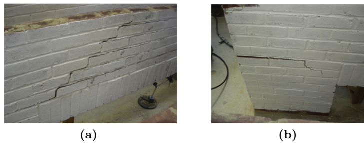
Figure 2.35. Damage observed in the experiment (Giamundo et al., 2014)
