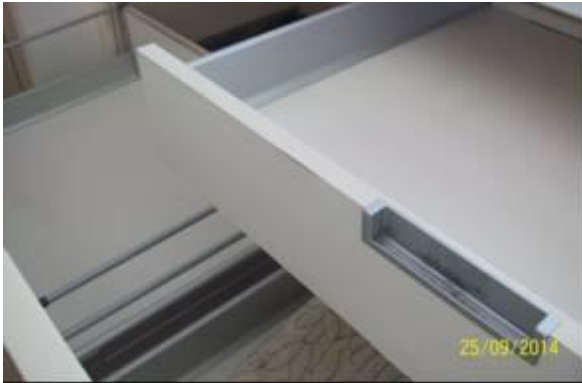
The drawers of the kitchen have wet damages.
