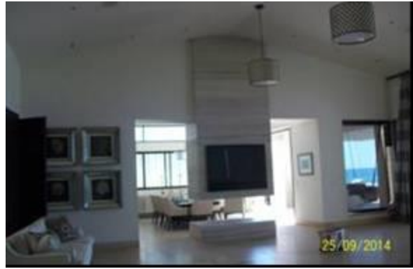
Living / dining rooms with humid ceilings.
