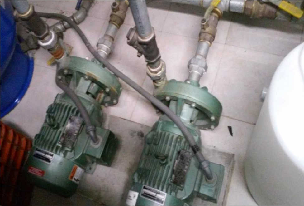
fig (6.11.12) bombas centrifugas
