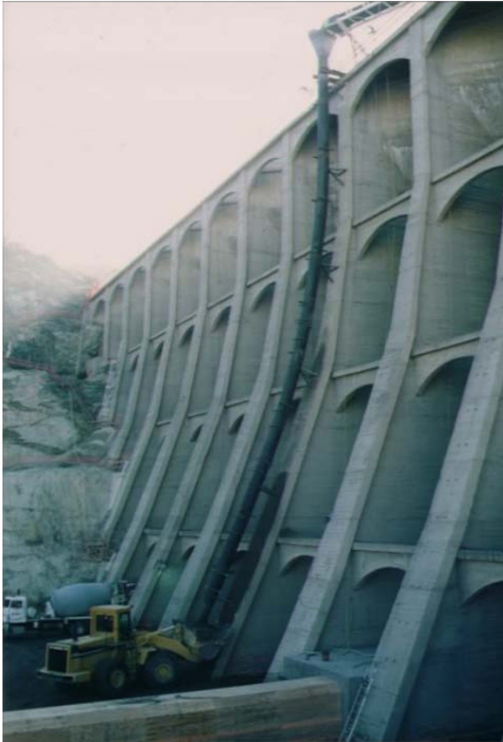
Figura 1- 23 Little Rock Dam California vista aguas abajo (Hansen K. , Rehabilitation of Existing Dams with RCC, 2008)
