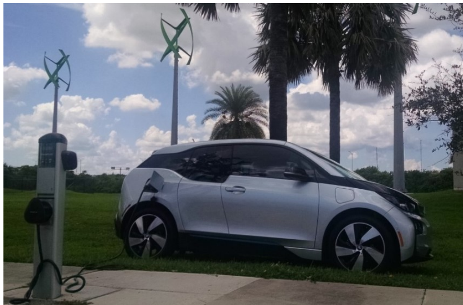
Photograph 4.19 Integrated Renewable Energy.
