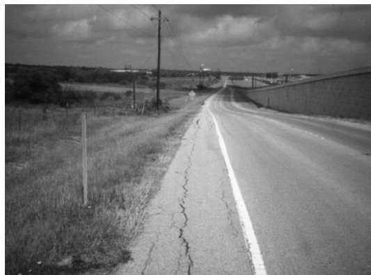
Fig. 2-8 Grietas laterales (Soil Stabilization of Oklahoma, s.f.)
