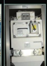
Common Cabin Air Assembly (CCAA) condenses water vapor from air.
