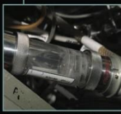
The Russian Condensate Water Processor is known as the SRV-K, equivalent to the US WPA, processes the condensate that is reclaimed by the SKV.
