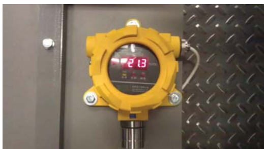
Figure 5.23: Oxygen detector - Reading from the Oxygen detector in a nearby lab.
