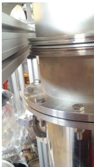
Figure 4.9: Transitory Connection - A pipe that will be replaced for a LF250 flexible nipple.
