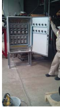
Figure 4.11: Power Facility - An image of part of the new electrical system to power the supersonic jet beamline.
