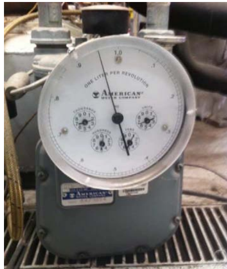
Figura 5.12 Medidor de gas American Meter Company.
