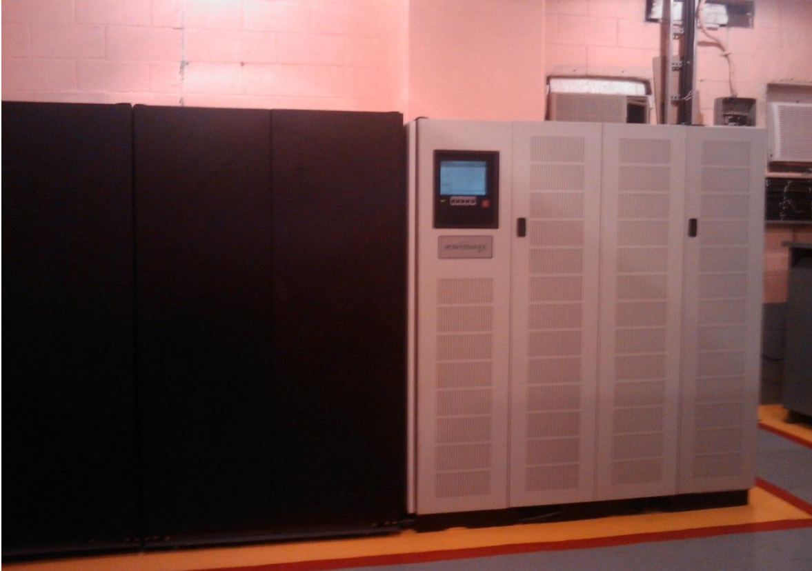
Figura 3.27 UPS ON LINE de 225 KVA
