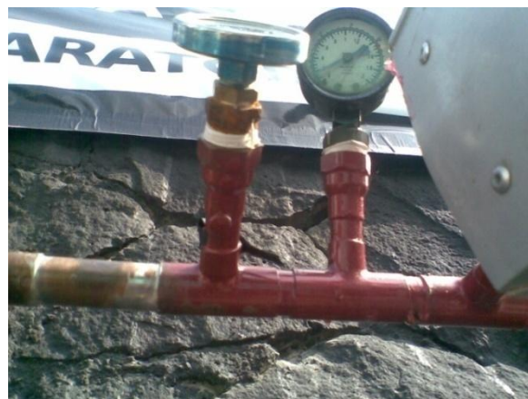
FIGURA 3.16. Colector Solar B.
