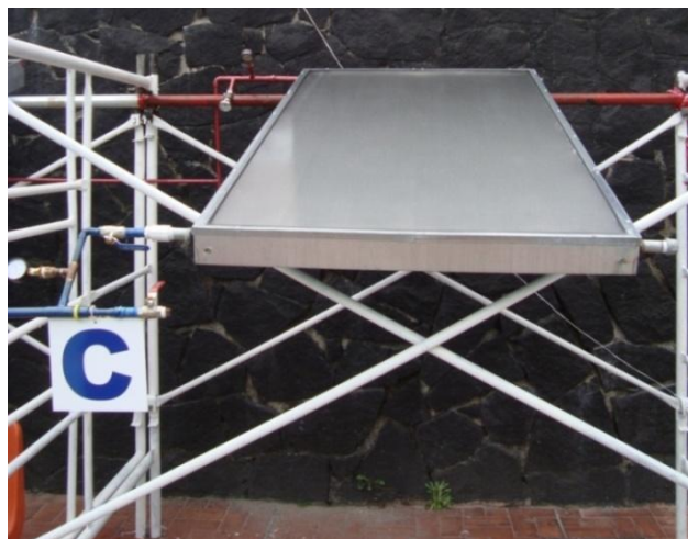
FIGURA 0.8 Colector solar "C"
