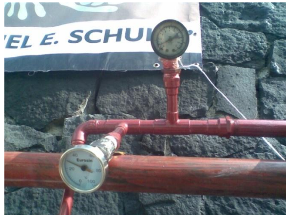
FIGURA 3.17. Colector Solar C.
