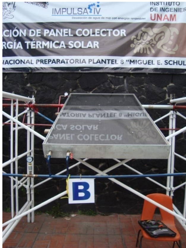
FIGURA 0.4 Colector solar "B"
