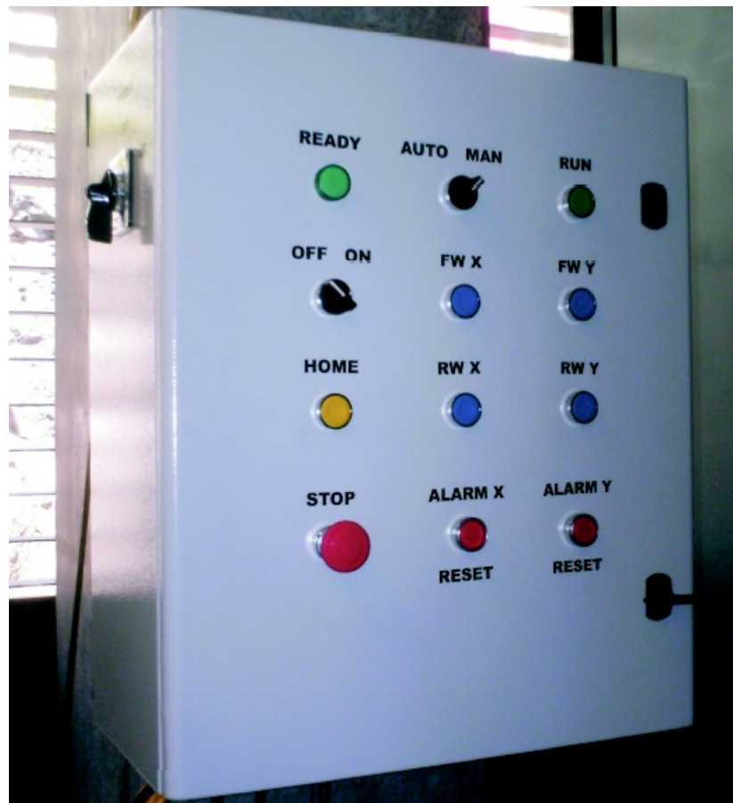
Figura 7.2: Panel de control
