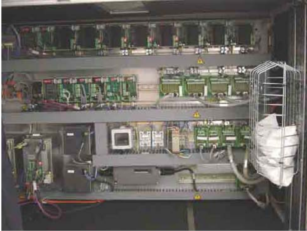
Figure 7: Electronics Cabinet inside view. Stepper motors controllers located at top. Temperature sensors, Shutter and calibration modules at the middle. Turntable and focusing stage stepper controller at bottom left.
