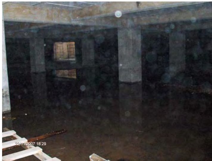
Figure 4: Cellar flooding in Díaz Infante Hospital building (January, 2008)
