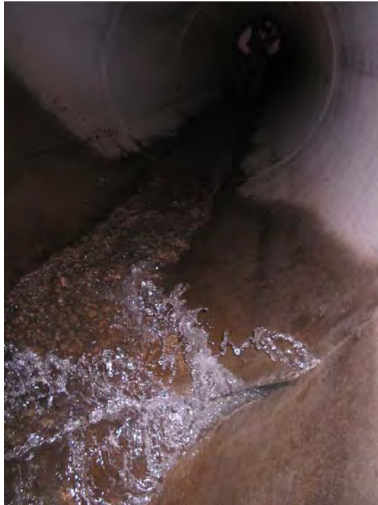
Figure 3. Groundwater infiltration in Hernán Cortés Stormwater collector (December, 2007)
