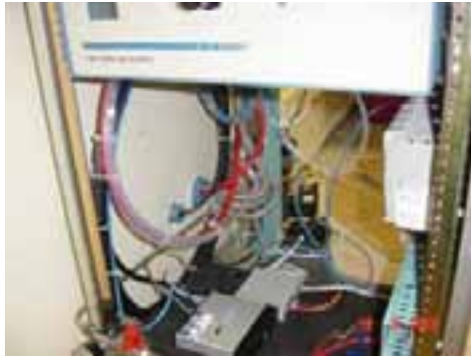
Figura 3.5. PLC Allen Bradley
