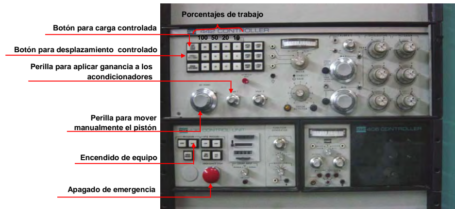
Figura 2.5 Tablero de control
