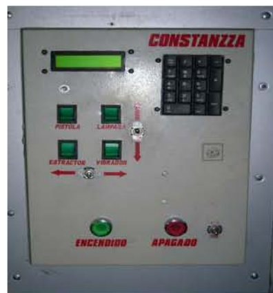
Figura 6.5 Panel de control
