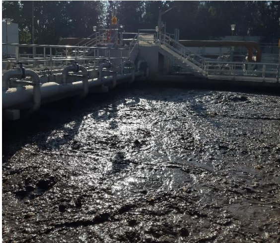
Figura 3.14. Reactor aireado, PTAR Chapultepec
