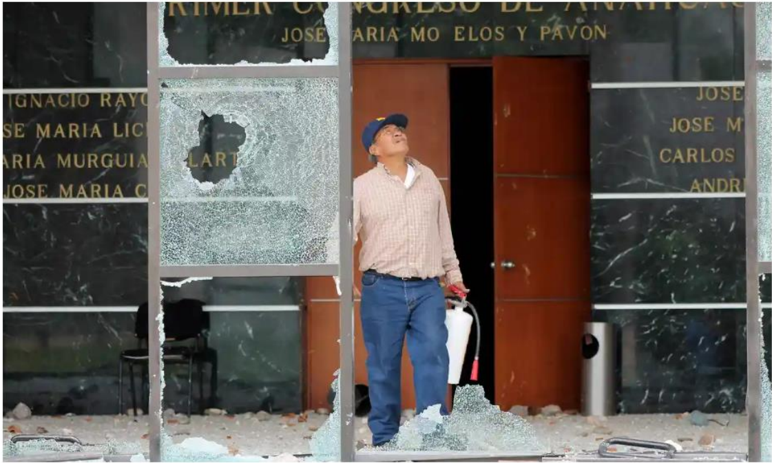
📷 A civil servant surveys damage at the Guerrero state congress building in Chilpancingo. Photograph: EDUARDO GUERRERO/AFP/Getty Images
