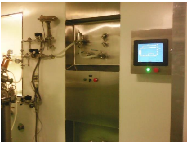
Img. 19 PLC UniStream
