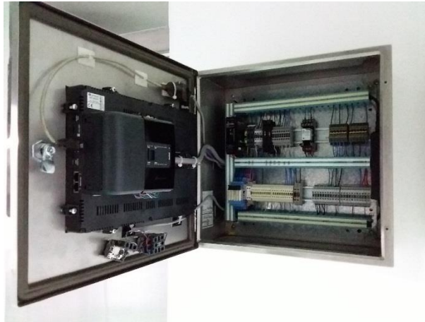
Img.65 Panel de control.
