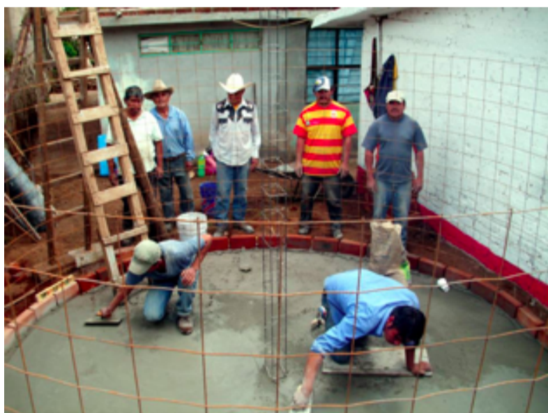
Image 4.2. Seven men participated in the cistern building capacity program with funding provided by the Monarch Butterfly Fund (MBF) and skills provided by Alternare June 2013 at the Alvaro Obregon Elementary School in Carpinteros. Several are shown polishing the cistern floor. One of the participants was quoted saying, “The rainy season has just started, and water collected in this cistern will be a valuable resource to this school during the dry season”. Photo provided by MBF.
