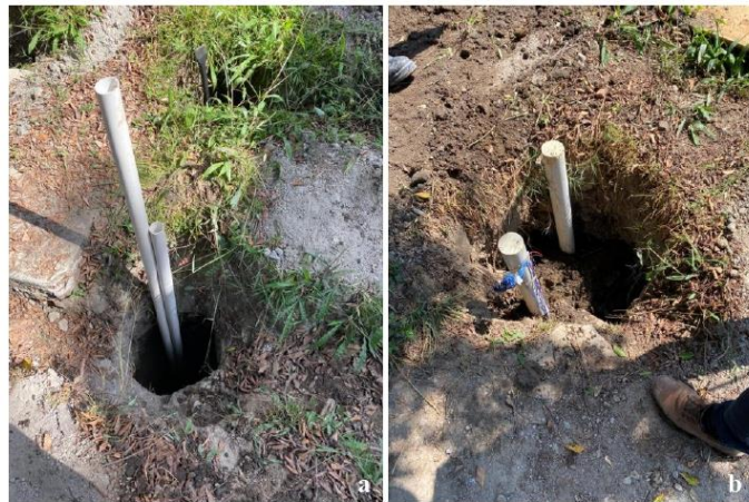
Figure 1: The figure above shows a) the pipe into the well, b) the well backfill with the pipe.
