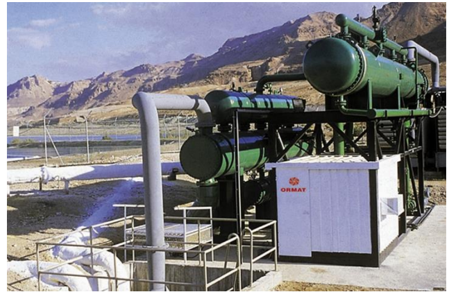
Figura 6. Ormat 150 kW (Bronicki, 2017).
