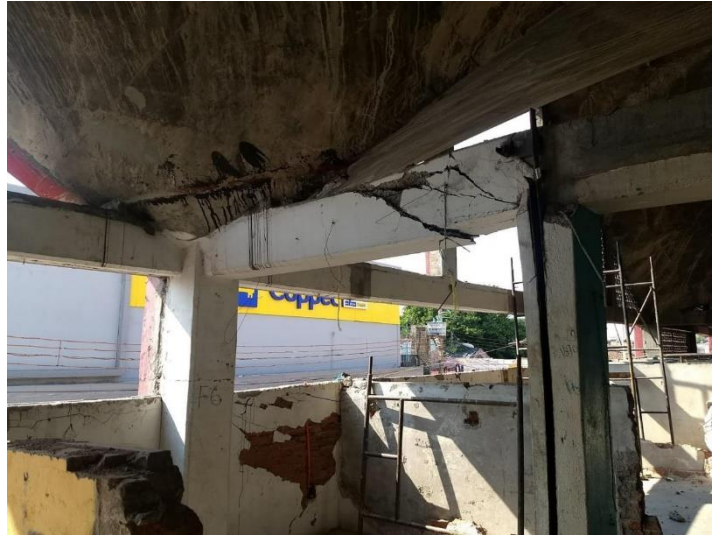
Fig. 4 Settlement in the Juchitán market property, which caused damage to the mezzanine
