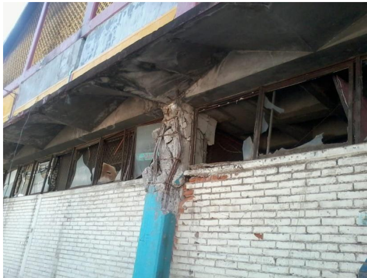
Fig. 3 Short column effect on columns of the Juchitán market building
