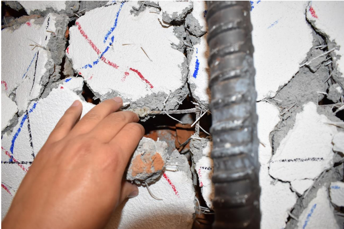
Figura 174. M-12R a \delta = 0.010 . Grieta pico: 6.0 mm, grieta residual: 2.5 mm.
