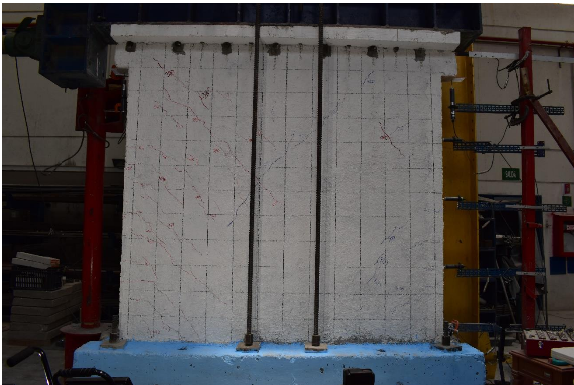
Figura 133. M-3R a \delta = 0.002 . Grieta pico: 0.2 mm, grieta residual: 0.1 mm.
