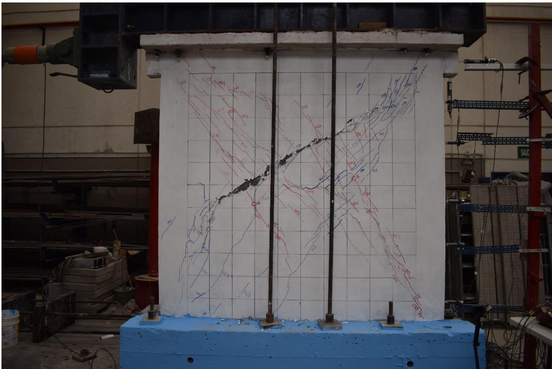
Figura 157. M-8R a \delta = 0.005 . Grieta pico: 1.5 mm, grieta residual: 0.8 mm.
