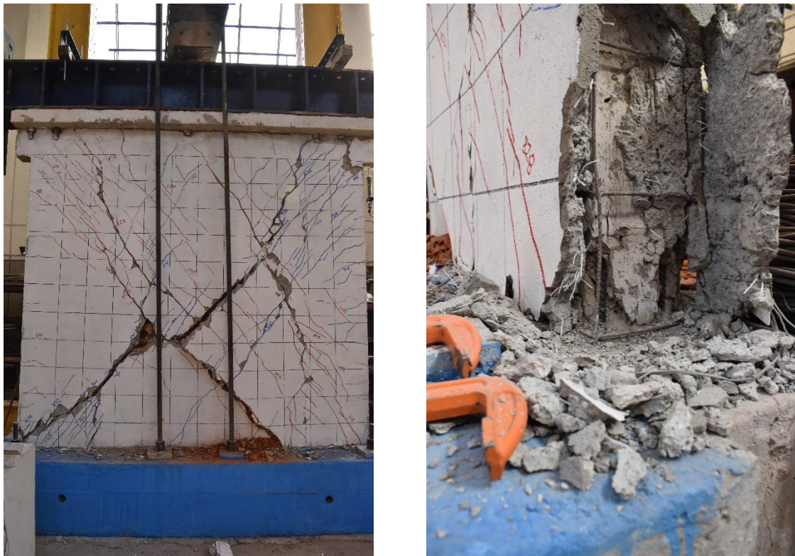
Figura 153. M-7R a \delta = 0.010 . Grieta pico: 30 mm, grieta residual: 20 mm.
