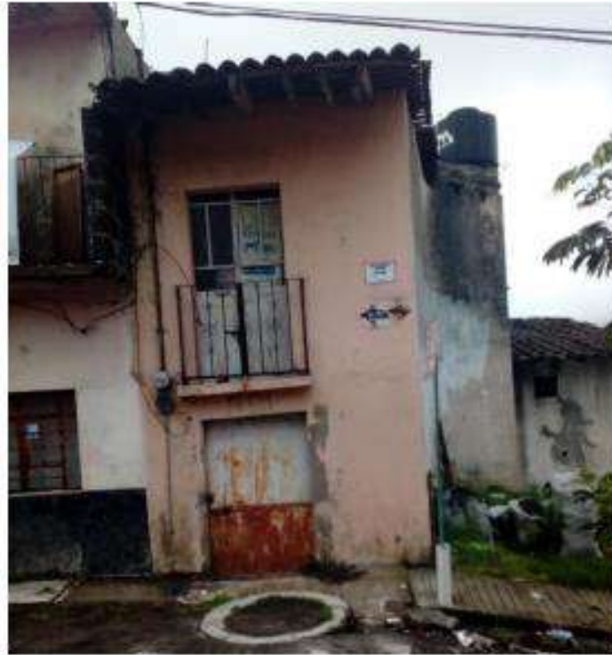
Fig. 3 Poor housing and unmanaged settlement construction on unstable slopes in La Gloria neighbourhood increase exposure conditions to landslides and other hazards.
