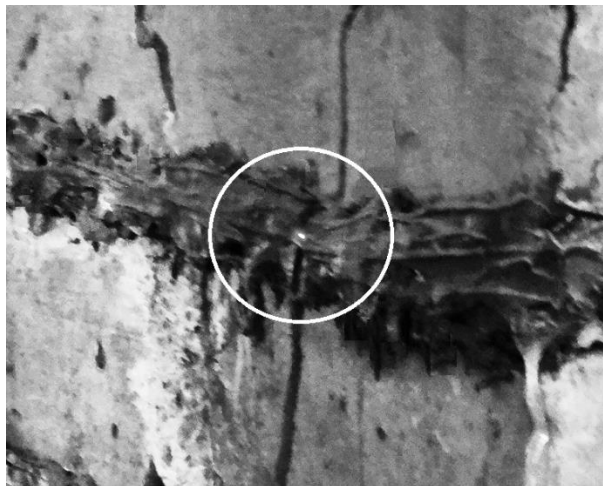
Fig. 1. The fracture and glow of the optical fiber, fixed with epoxy adhesive on a brick wall, due to the appearance of a crack in it (photo).
