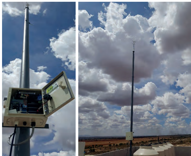
Figure E.4 Final installation of the WindMaster datalogger.
