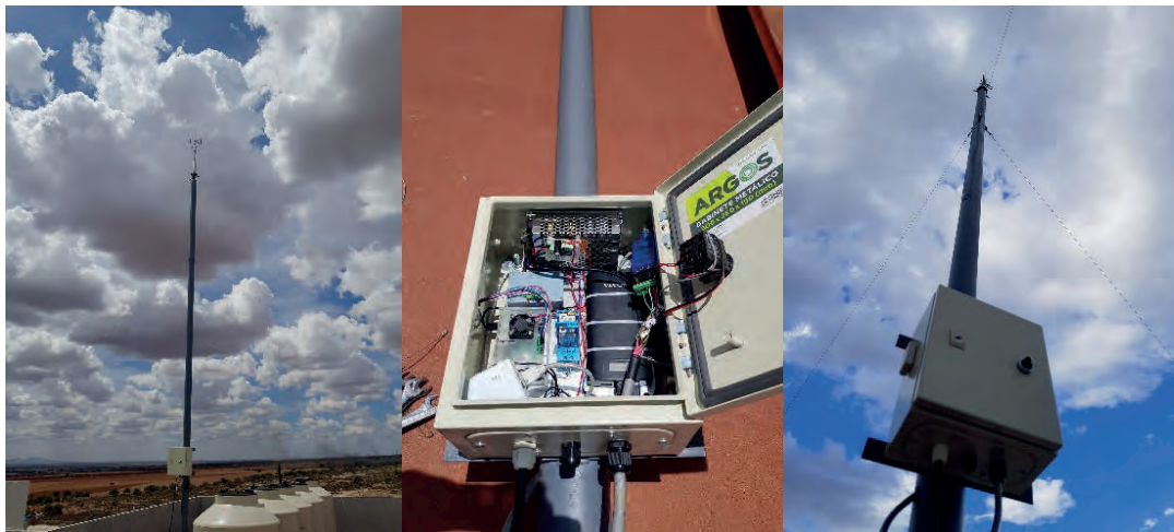
Figure E.7 Final installation of the WindMaster ultrasonic anemometer.
