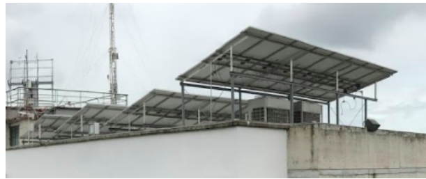
Figure 2.17: Photograph of photovoltaic system in Building 3.1.
