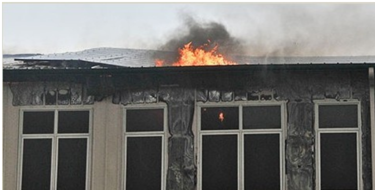
Figura 9. Incendio en la sede corporativa de Organic Valley en La Farge. En “Perfect Storm” , por Robert Duval, 2014. Recuperado de https://www.nfpa.org/News-and-Research/Publications/NFPA-Journal/2014/January-February-2014/Features/Perfect-Storm . Copyright [2014] por National Fire Protection Association.
