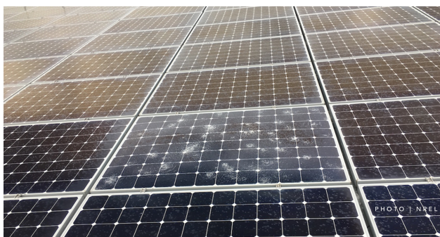
Figura 22. Módulo dañado debido al granizo. Recuperado de https://www.energy.gov/ee/articles/hail-no-national-labs-solar-panels-survive-severe-storm . Copyright 2018 NREL.
