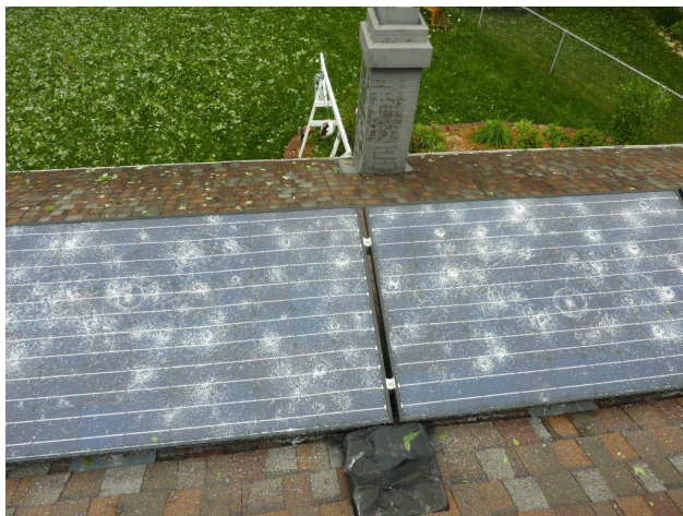
Figura 21. Módulos dañados en Maryland Heights. Recuperado de http://forum.solar-electric.com/discussion/14316/solar-panel-damage-from-hail-storm
