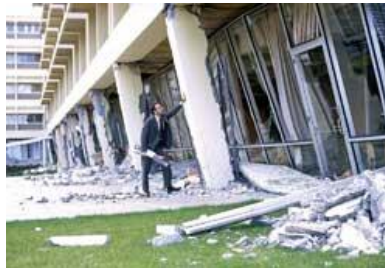
Figura 2.48 Hospital Olive View 3
