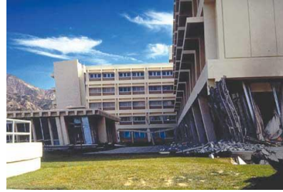
Figura 2.47 Hospital Olive View 2
