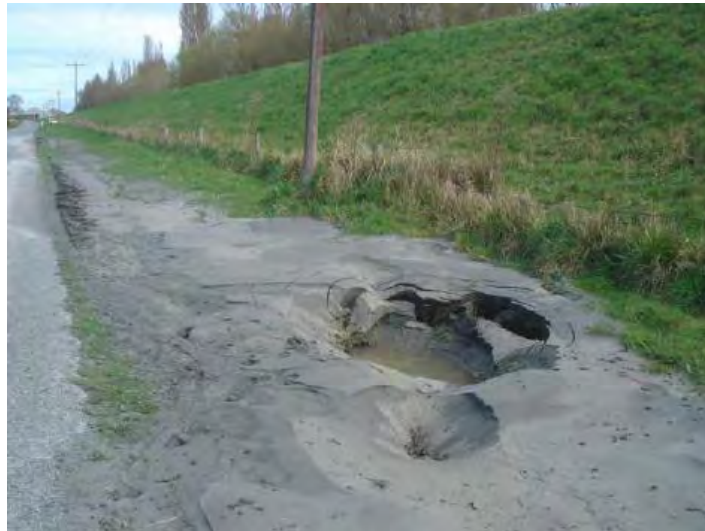
Fig 1.3 Gran volcán de arena en la base de una ladera (Geo-engineering Extreme Events Reconnaissance Association [GEER Association], 2010c)
