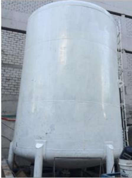
Fig. 2.38, Tanque Vertical 35 m 3
