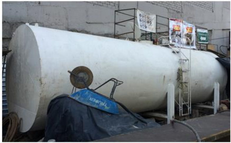
Fig. 2.39, Tanque Horizontal 30 m 3
