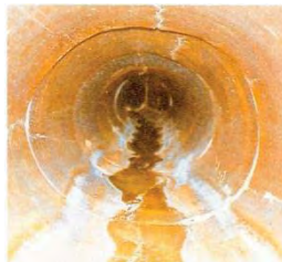
Figura A.277a – Tubo defectuoso
