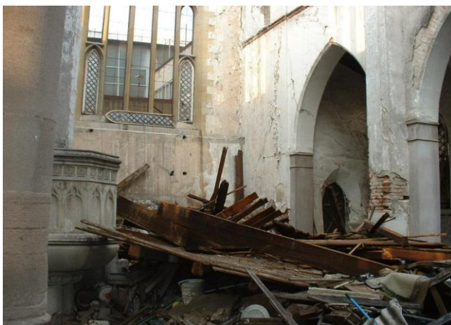
Foto43, desplome del techo de Christ Church,
