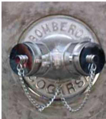
Figure 4.50 SFT Fire Fighting system of the Gulf of California (cogarsa)
