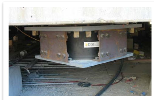
Figura 2.15 Utah State Capitol's Isolator
