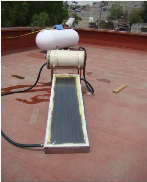
COLECTOR SOLAR INSTALADO
