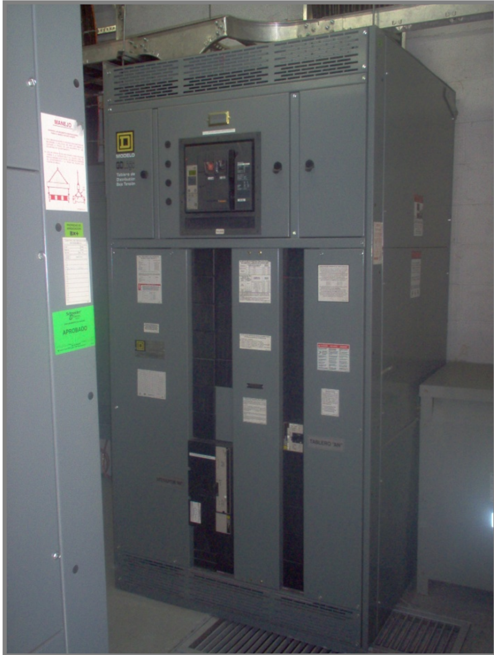
Figura 8.5 Tablero General Principal.
