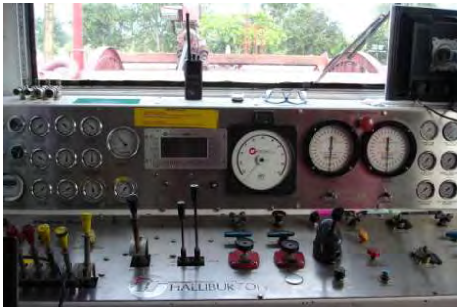
Fig. 2.6. Panel de control
