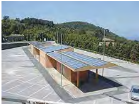
Car park installation (Courtesy: SEI, Italy)
